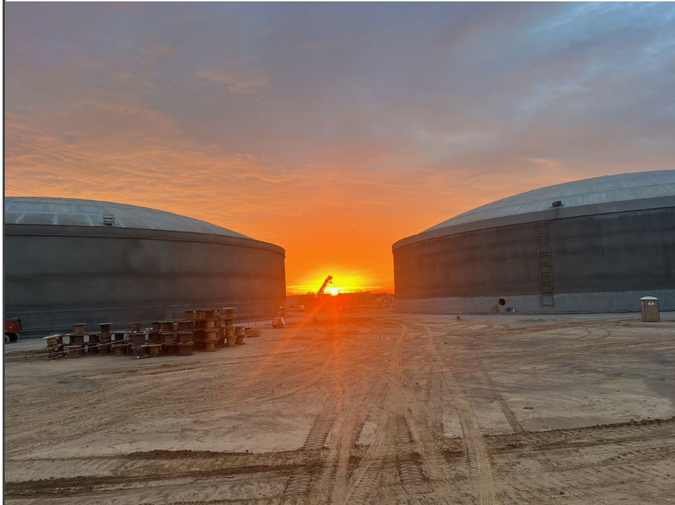
SWSP Central Pump Station at Sunrise
