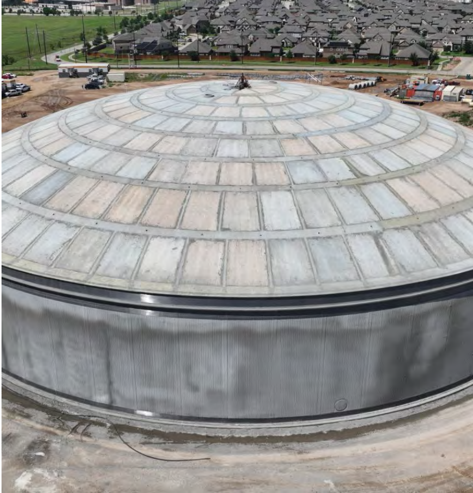
Central Pump Station – June 2024
