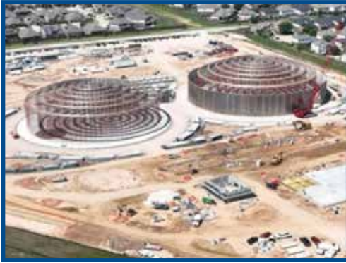
Central Pump Station (March 2024).
