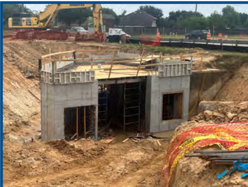
CPS Stormwater Junction Box
