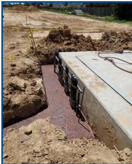
C1 Butterfly valve vault
