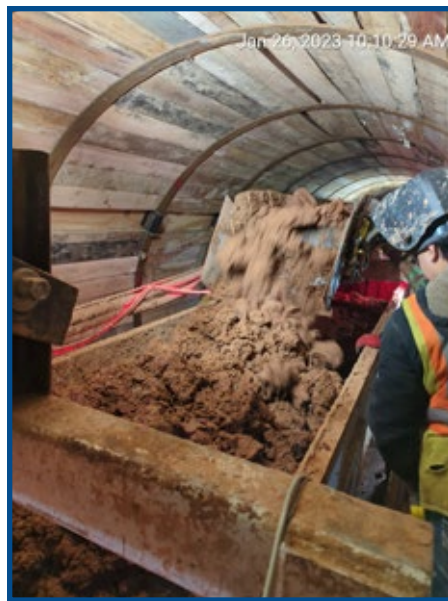
B3 Conveyor Within Tunnel
