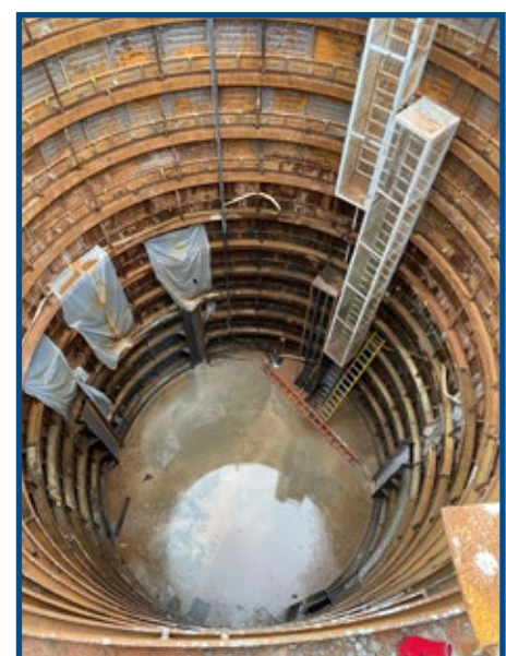
B3 Shaft at Site 2
